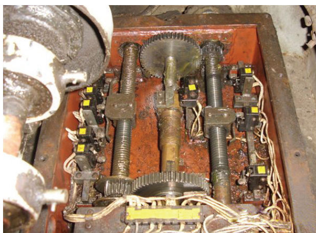
Limit switch cover missing
