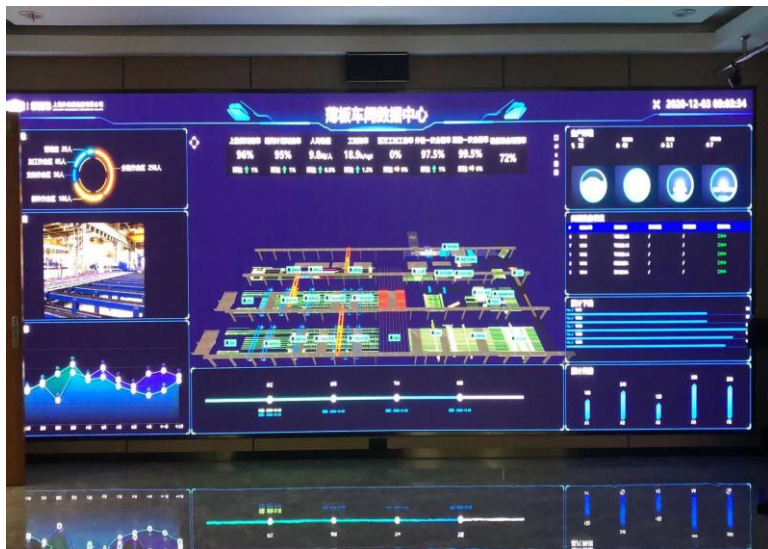
Intelligent Energy Management and Control System Panel
