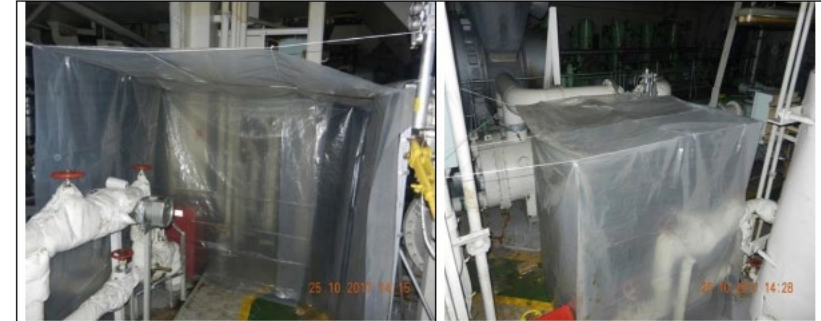
Enclosure Room from outside
